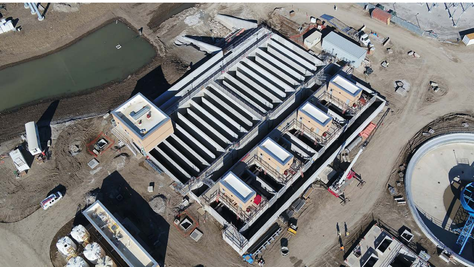
Filter and disinfection complex, March 1, 2021
