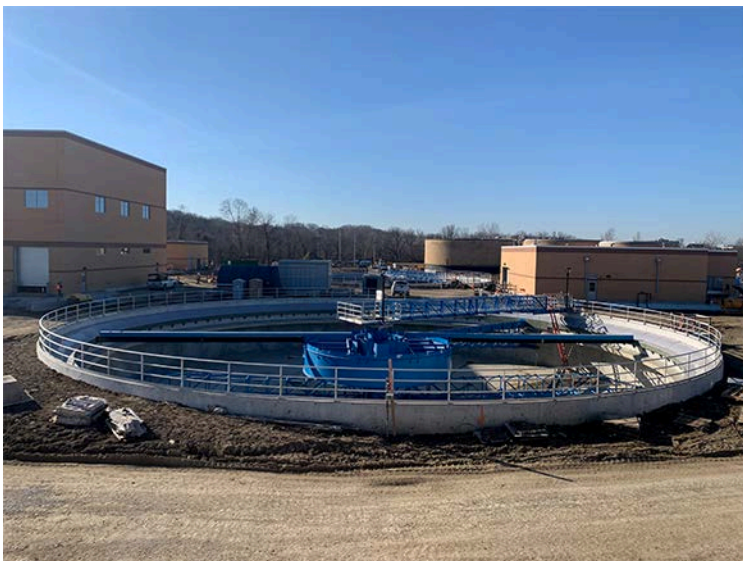
Final clarifiers at ground level, March 4, 2021
